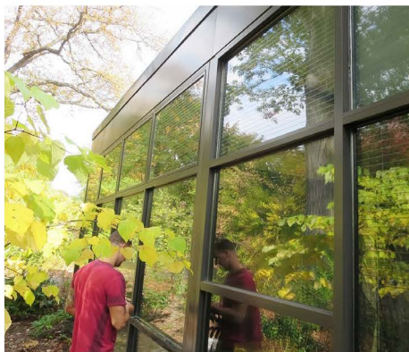
Solyx Bird Safety film covers the entire glass surface of this building at the Bronx Zoo. Photo: Chris Sheppard
